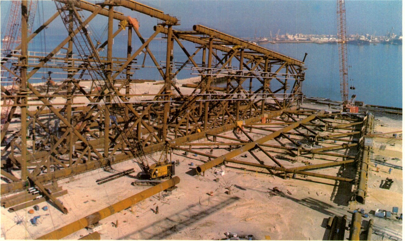
The platform jacket is being fabricated at Cadiz in Southern Spain. The jacket, as pictured above, is approximately 50% complete with four of the eight legs in their "rolled-up" position. Upon completion, the jacket will be skidded directly onto a barge for tow-out to location. Noting the comparative size of the workers in the picture gives some perspective to the size of the 8,000-ton structure.
