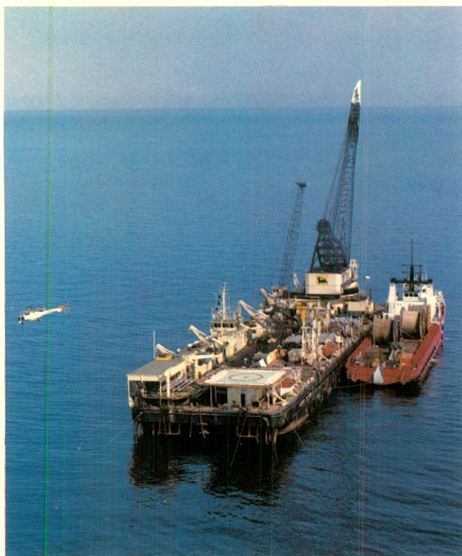
In October 1980, the 12" pipeline from the Afortunada to storage facilities at Tarragona was placed in service. This line was installed by the Castoro II lay barge shown above operating in 394 ft. of water, approximately 15 miles offshore.
