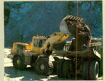
Ore is carefully handled by front end loaders for transportation to primary crusher.
