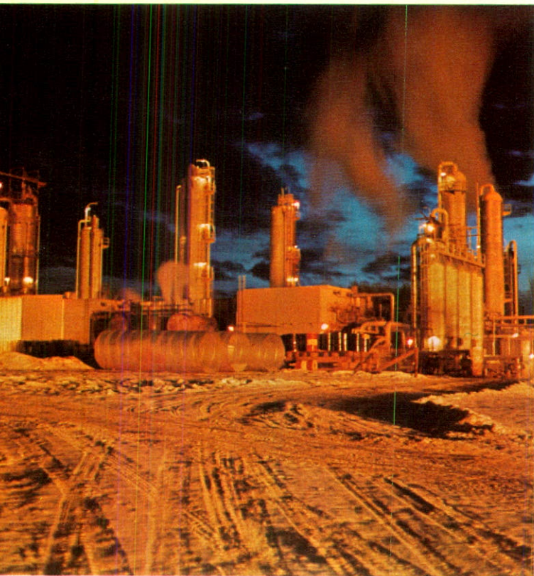
Westcoast's plant, near Fort Nelson, British Columbia, is the northernmost operation of its kind in the world, and is one of the largest gas-processing facilities in North America.
