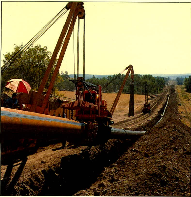
Upgrading of the mainline in the Cariboo district of British Columbia. Pipe with thicker walls replaces older sections to strengthen the system in an area where increased public activity is anticipated.
