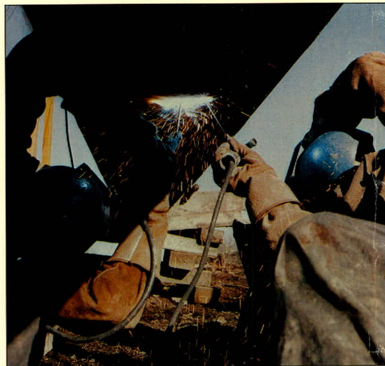
The welders' keen eyes concentrate on crucial joining of steel pipe sections.
