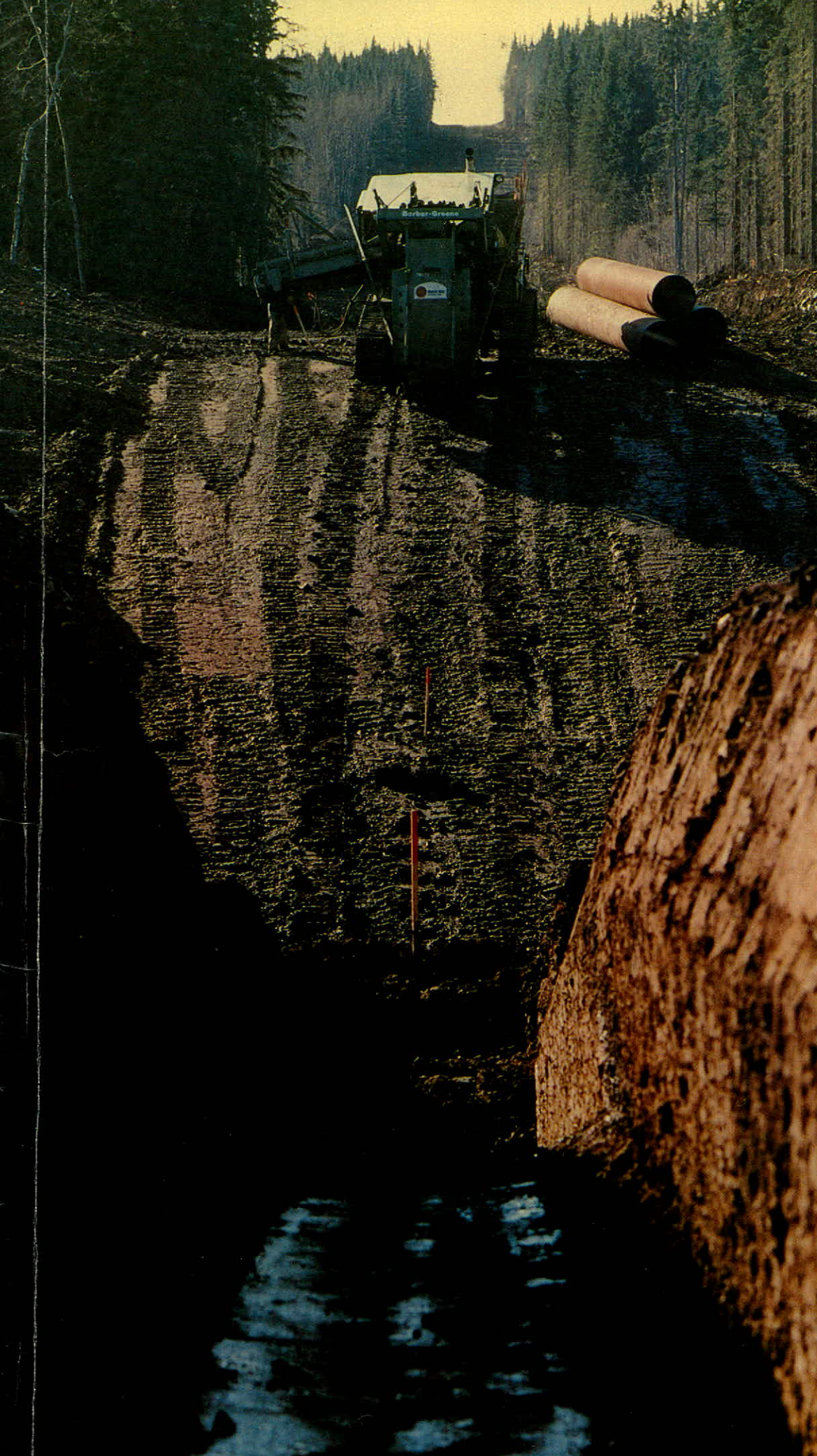
Pipeline trenching in the rolling forest lands of east-central British Columbia. Yawning trench in foreground is ready to receive pipe. Ditching machine at top centre prepares to extend the trench.
