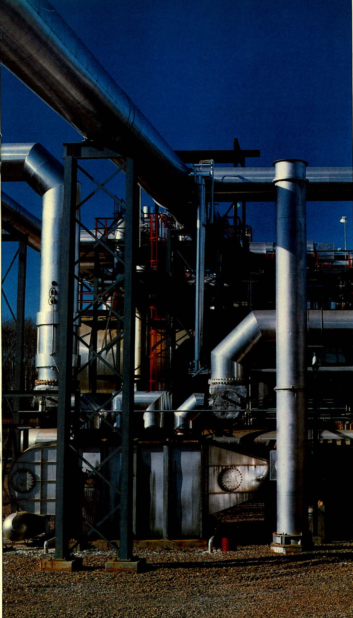
An intricate web of pipe in the Fort Nelson sulphur recovery plant.
