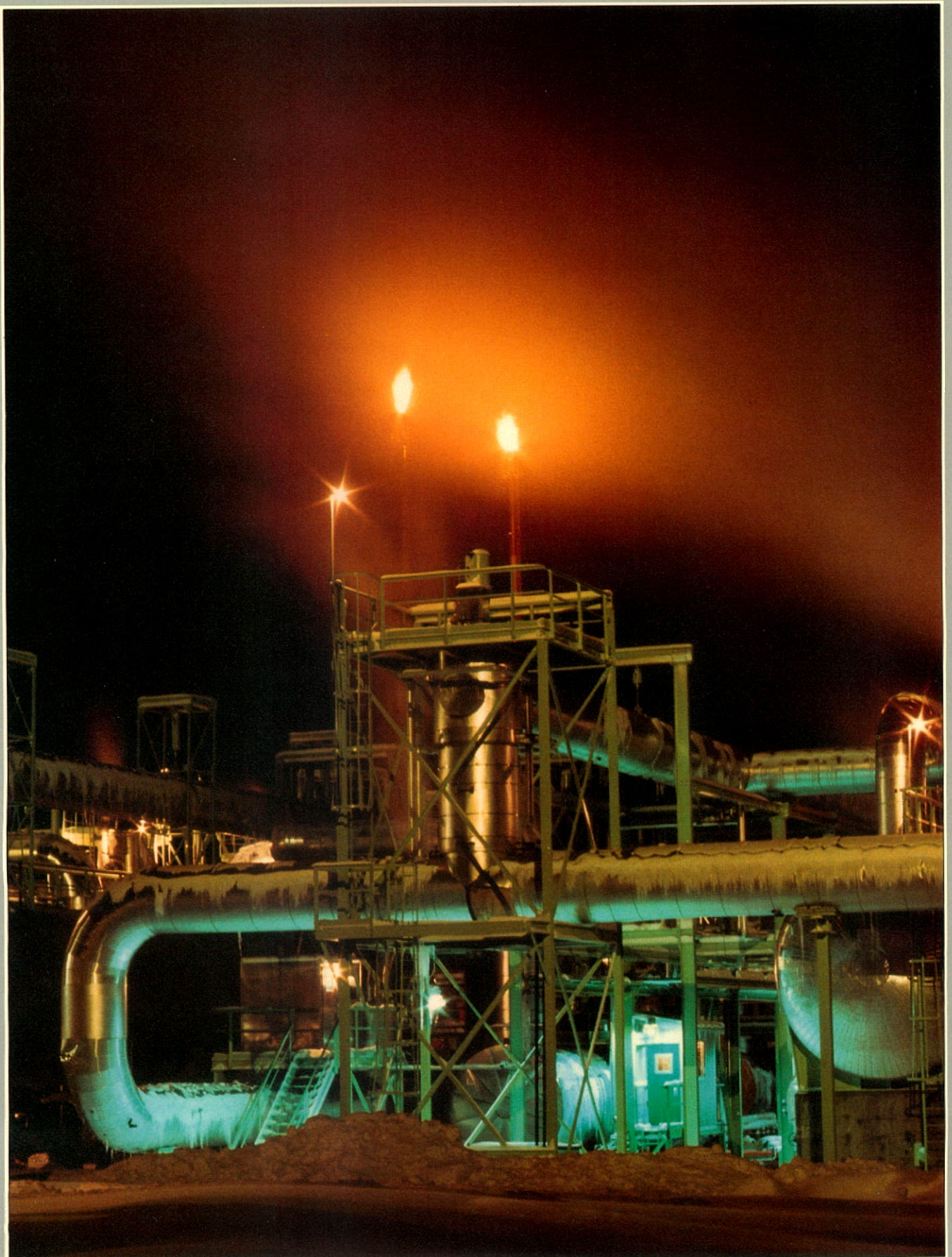
Sulphur Recovery Facility at Pine River Gas Processing Plant
