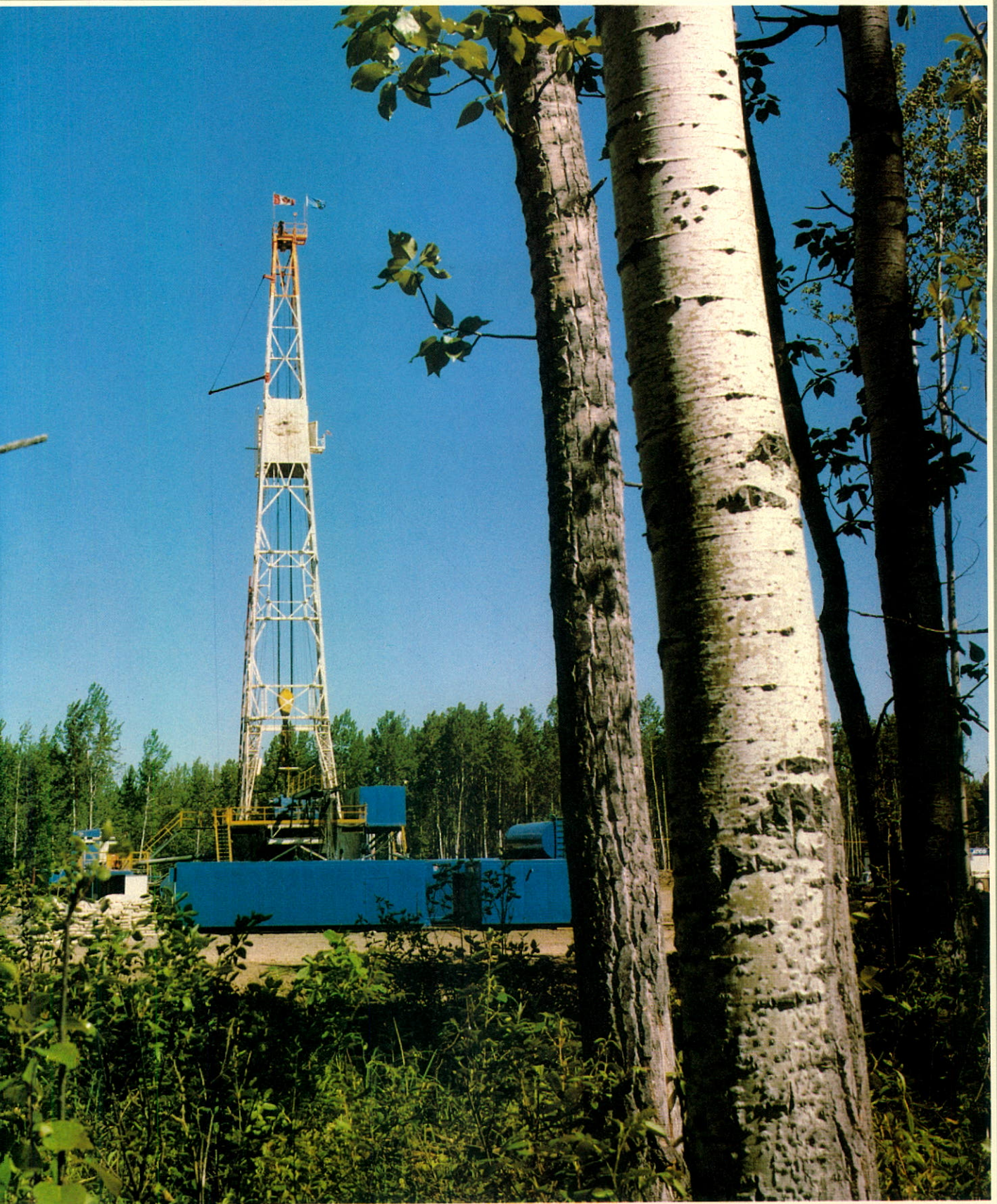
Canadian Hunter-Bluesky et. al., well drilling in the Elsworth gas field of western Alberta.
