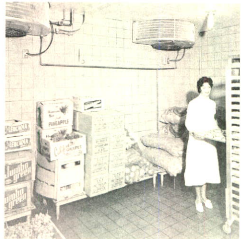
Bohn Half-Rounds control temperature and humidity, keep vegetables temptingly fresh in a supermarket walk-in cooler.
