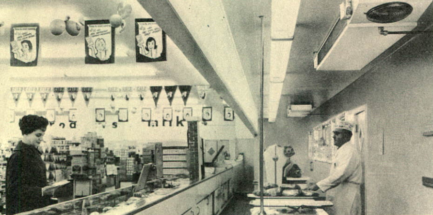
Bohn Unit Coolers are available in a wide range of models and sizes, complete with automatic defrost system. Shown here is refrigeration unit installed in meat-wrapping area of a national supermarket.
