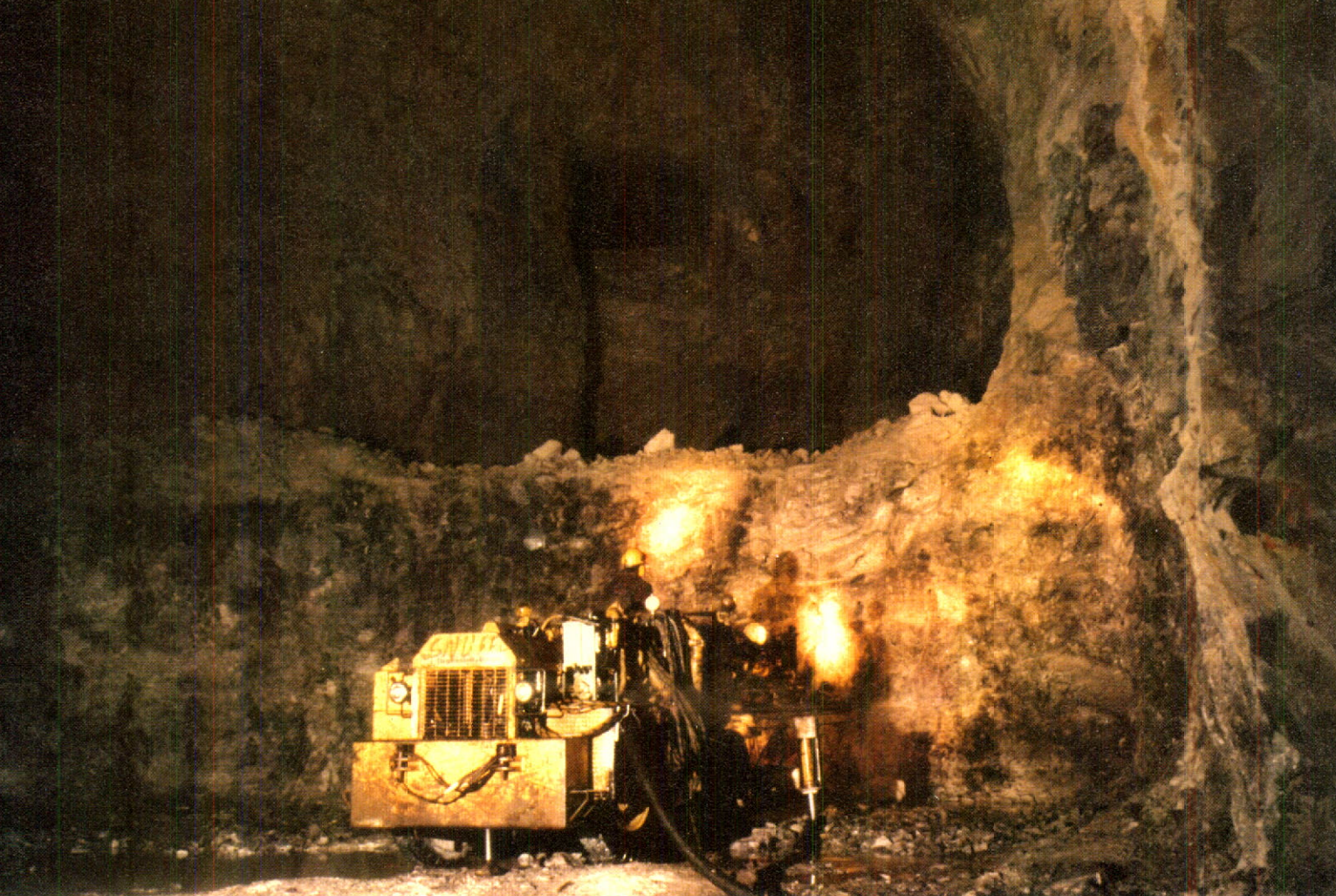
A two-drill jumbo drilling machine working in one of the many cavernous stopes at Tantalum Mining Corporation
