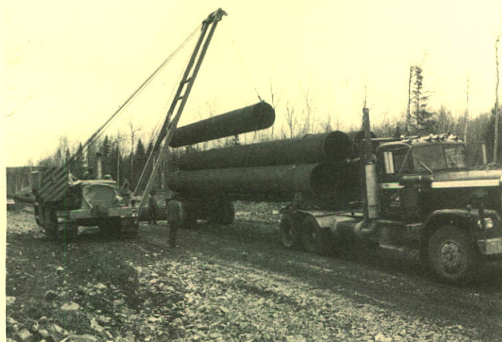
Stringing of 36" O.D. pipe during construction of looping facilities on a major Canadian pipeline in Eastern Canada.
