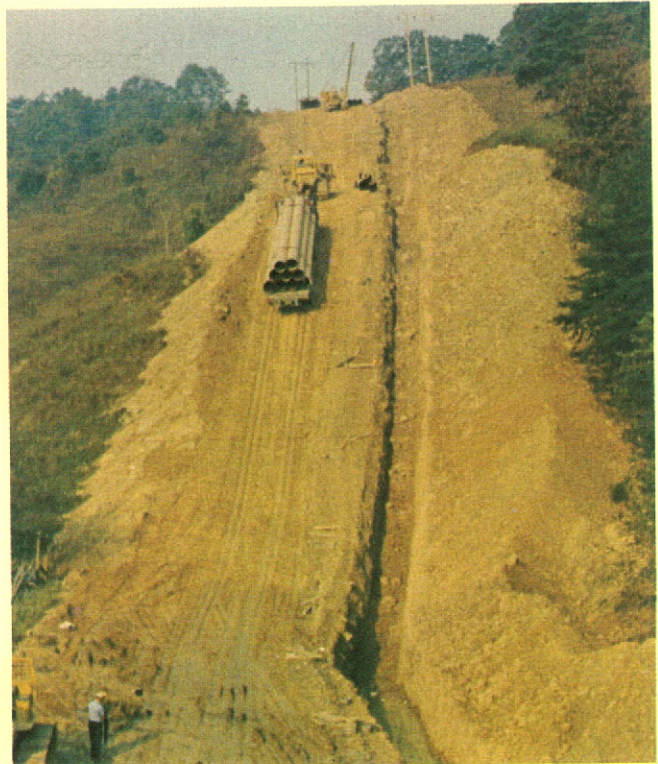
One of the company trucks being towed up a steep grade during a pipeline construction project in Kentucky, U.S.A.
