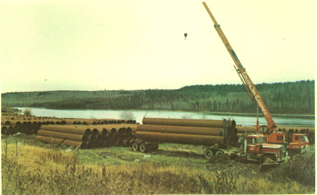
A truck being loaded at a stockpile yard prior to hauling the pipe to the right of way for stringing.
