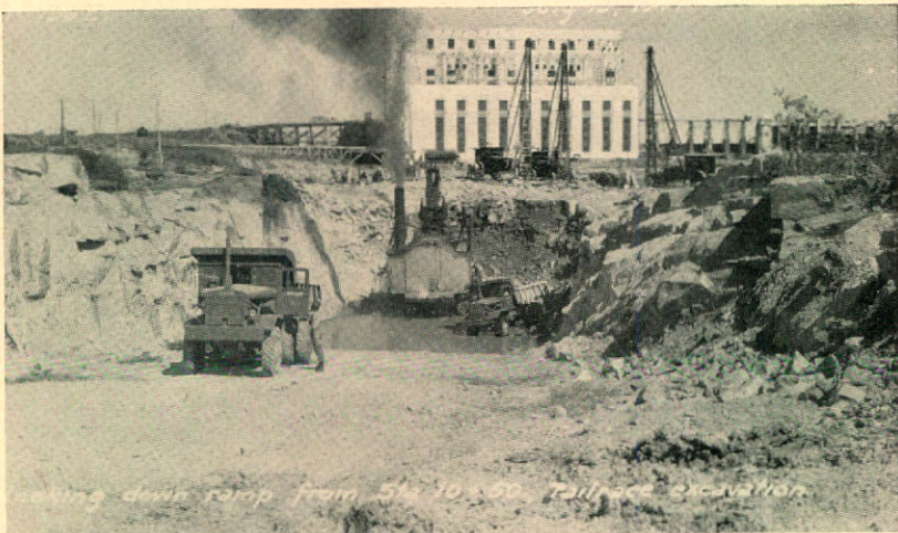
Lowering down ramp from 5 1/2 to 500' fall at excavation. Seven Sisters Falls: Removing rock from riverbed to deepen and extend tailrace.
