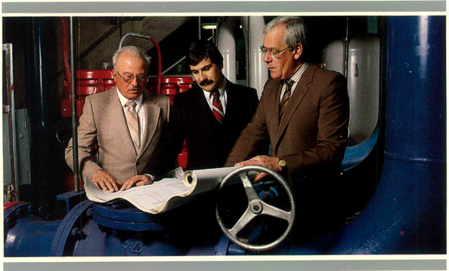
Trizec's Western Canada Operations Division: (from left to right) Tom Allen, Manager, Energy Conservation & Preventative Maintenance; Peter Kasian, Leasing Manager; Bill Elliott, Vice President
