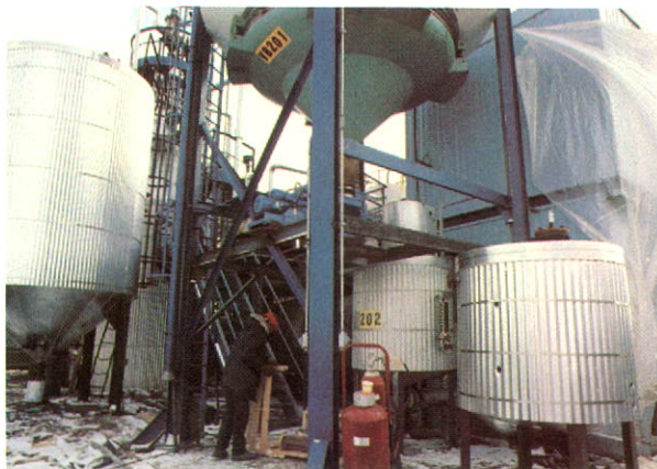
Pre-treatment Filter Press Equipment — Edmonton, Alberta
