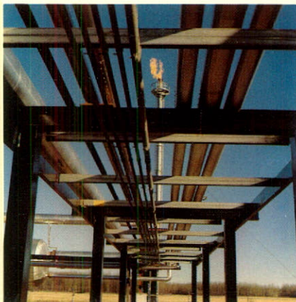
Wapiti Gas Plant flow lines.
