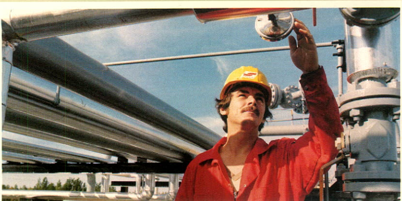
Operator making a routine tour at the Wapiti Gas Plant.
