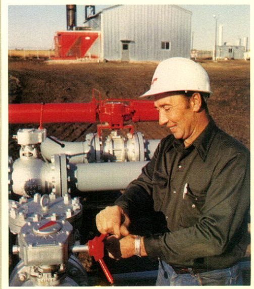
Senior Operator adjusts gas flow to the Plant.
