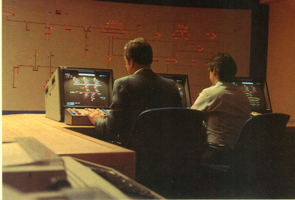
Ultra modern computerized control of its electrical system leads the Company into its second century of service.
