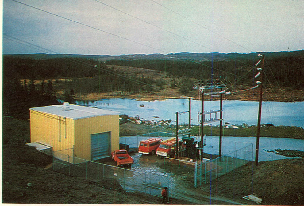
The 1,100 kW Morris Development located south of St. John's is the first new hydro energy source built by the Company in twenty years.
