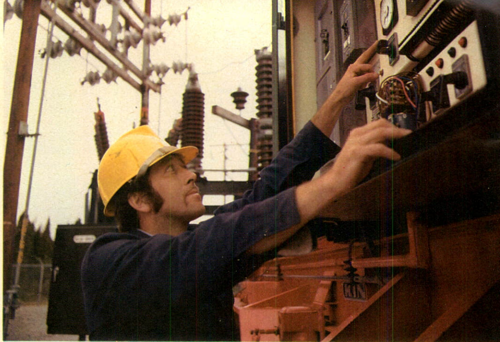
This mobile transformer at Gander shows specialized equipment responding to unusual electrical system conditions.
