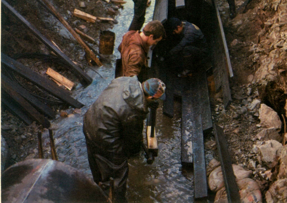
Woodstave pipes such as this one at Topsail are like long barrels and require special construction skills.
