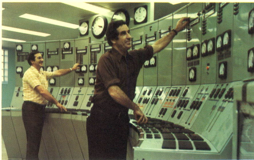
Constant monitoring of the electrical system at control centres helps maintain a high level of service.
