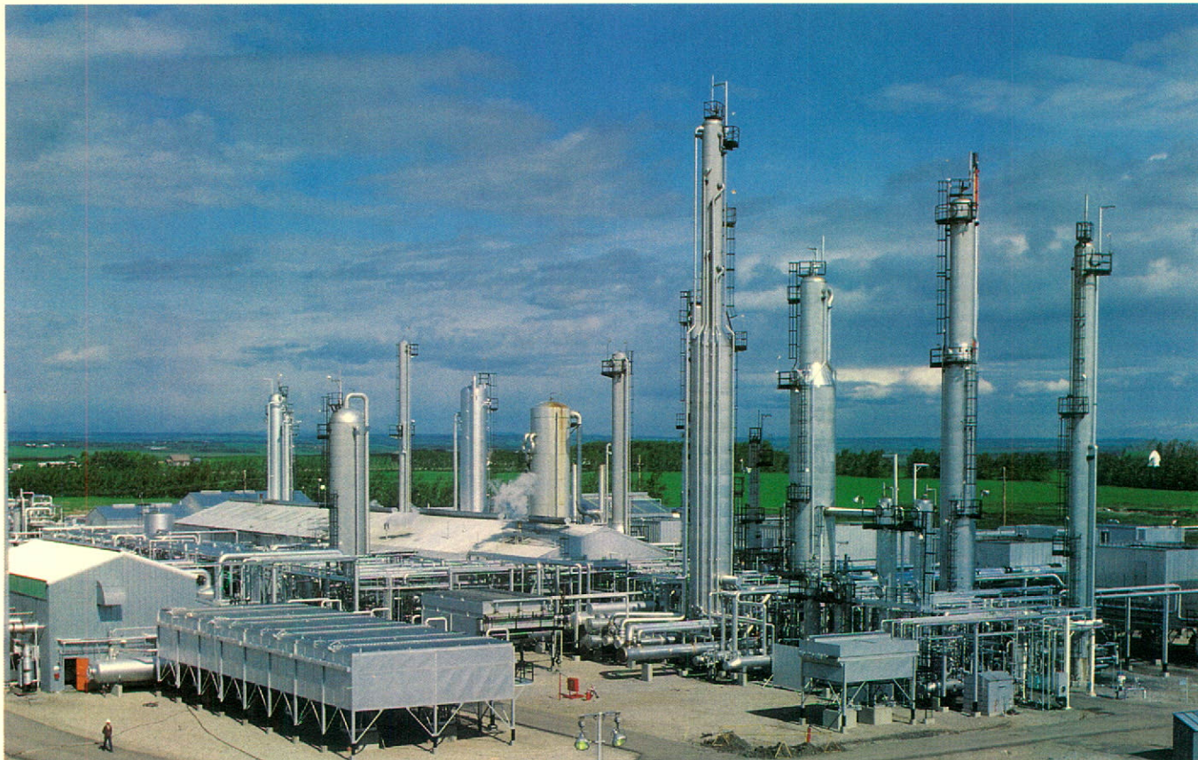
Processing area at the Carstairs, Alberta natural gas processing plant.
