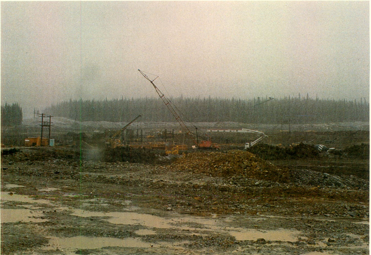
Snow and rain in mid-June slowed construction by making some areas impassable for heavy vehicles.
