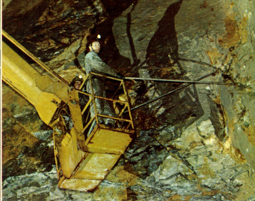
A miner, working from the platform of a Giraffe, scales a face after a blast. Jersey Mines.
