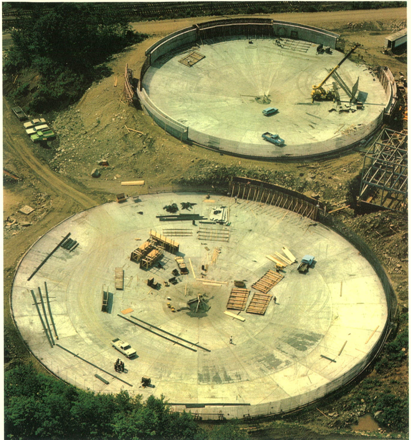
Wastewater clarifier tanks under construction at Brown's pulp and paper mill (right) are a key part of the major pollution control project at this New Hampshire facility.
