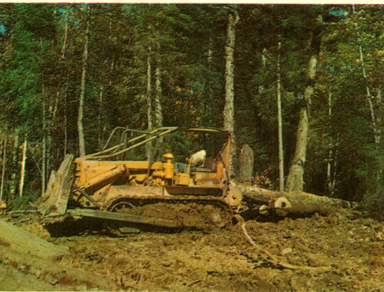
Crawler type tractors serve a dual purpose in woods operations. Equipped with blade, they can clear and build woods roads. They possess the needed power to ground-skid, and log with sulkies, tree length hardwood timber to central yards where it can be graded and cut to most profitable lengths for veneer logs, sawlogs, boltwood and pulpwood.
