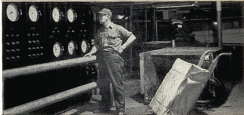
1950 The Riverside Paper Mill was modernized with the installation of a new hydrafiner and pulper with automatic controls. Also, many improvements were made to increase mill efficiency and to reduce pulpwood costs.
