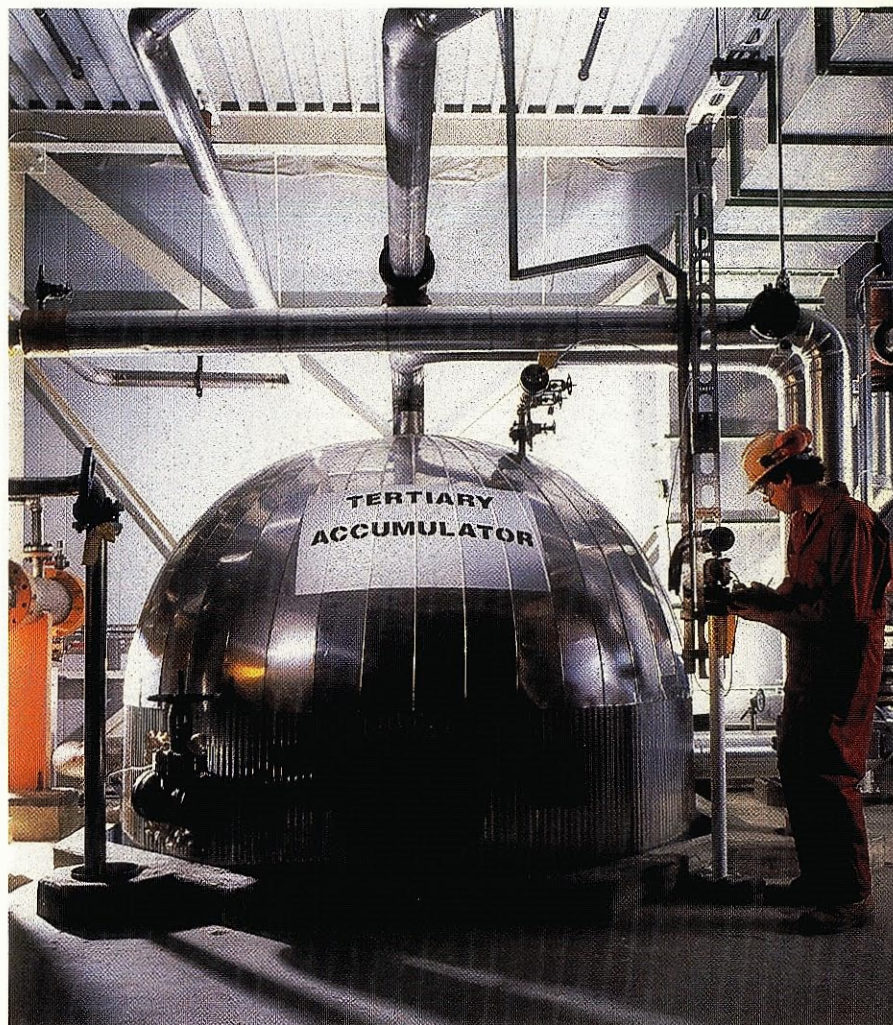
TERTIARY ACCUMULATOR HOLDING FRESH LIQUOR FOR EXTRACTION.
