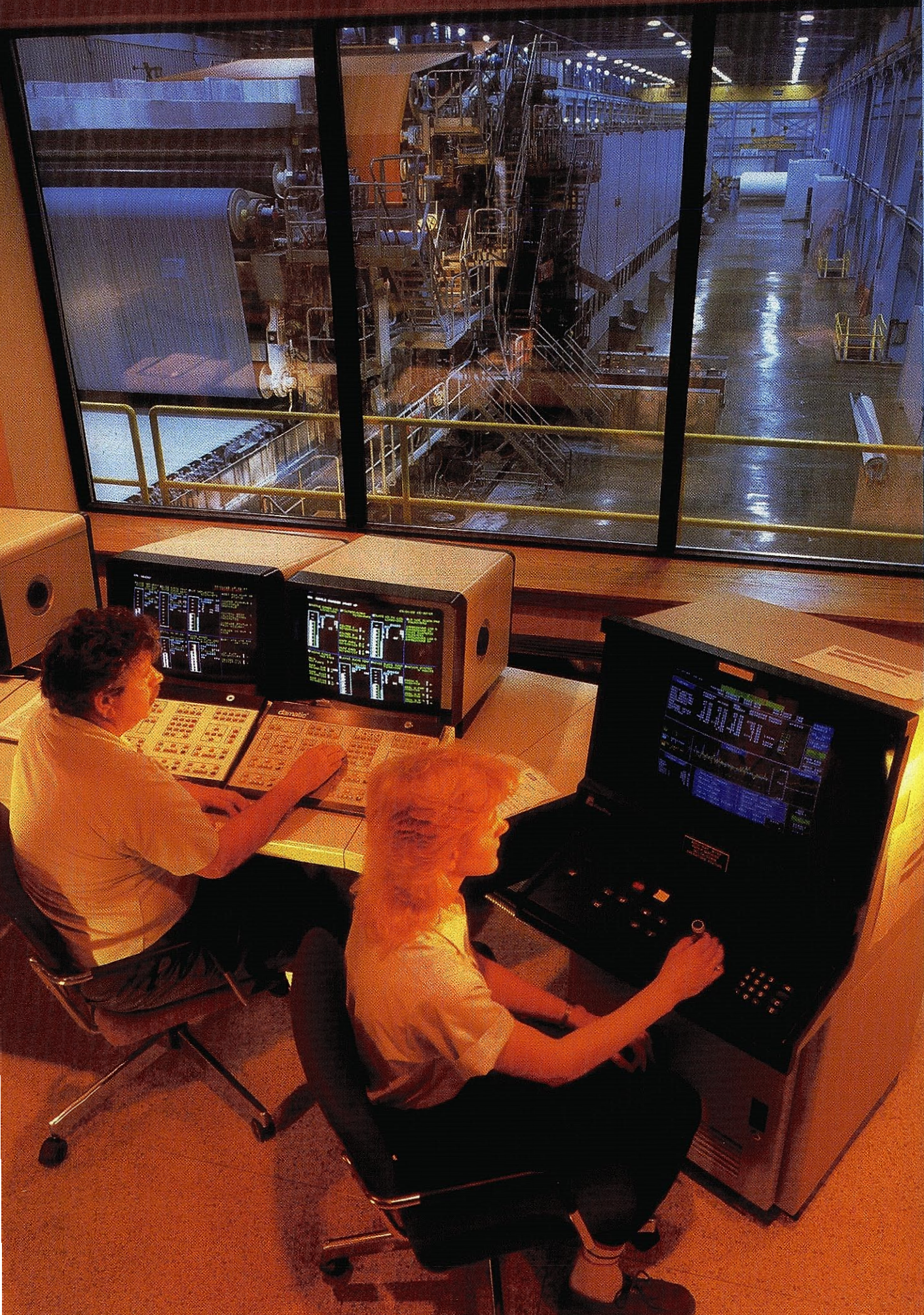
CONTROL ROOM OVERLOOKING M-7
