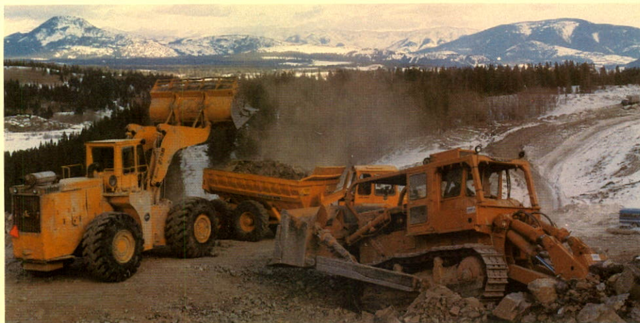
Regular blasting and quick follow-up loading characterized this mountain road building job. Loading chores were assigned to a Clark Michigan 275B, with a Komatsu D155A assisting on ripping boulders.
