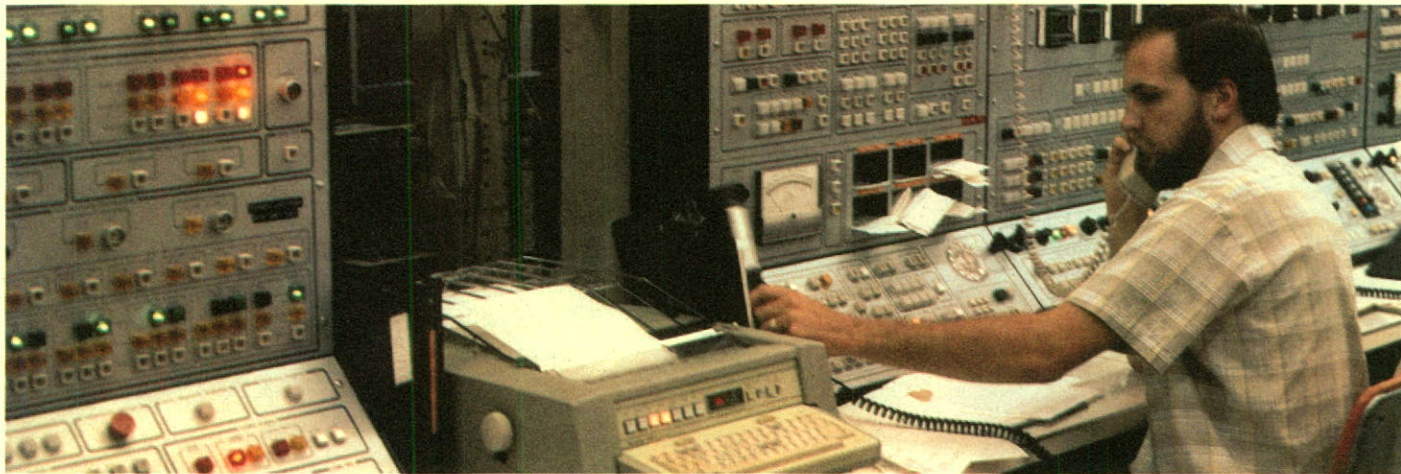
A Stored Program Control (electronic) console
