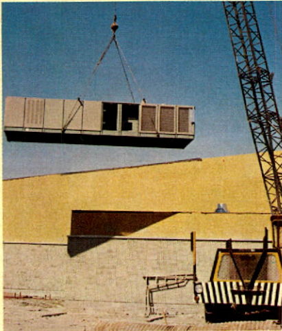
Installation of a Flame-Master roof top heating unit
