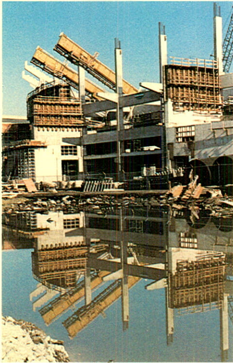
British Columbia Place under construction in Vancouver. Our subsidiary Lafarge Concrete Ltd. has supplied 49,684 cubic metres of ready-mix concrete for the project.
